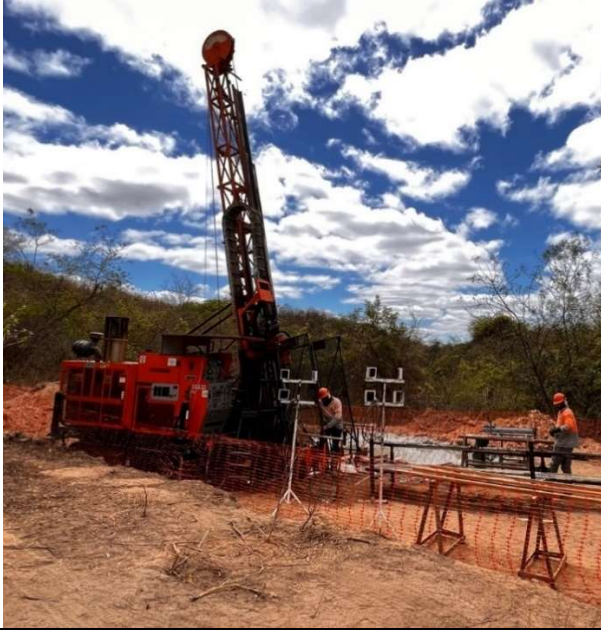
Drill Rig on site of the Bandeira, drilling in 13/09/2023 the DDH ITDD-23-192 - azimuth 140 – dip ~70
