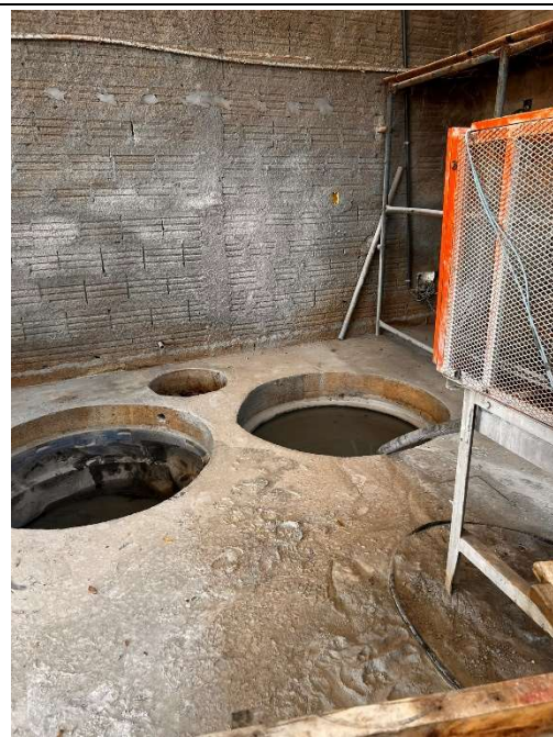
Drill core cutting saw sediment settling tank.
